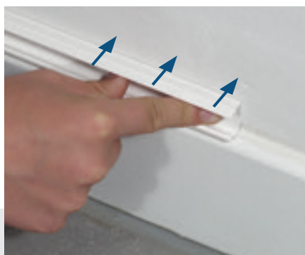
2 Place the mini-trunking in the required position and press it firmly against the wall. The thickness of the adhesive foam compensates for any flaws in the wall.
